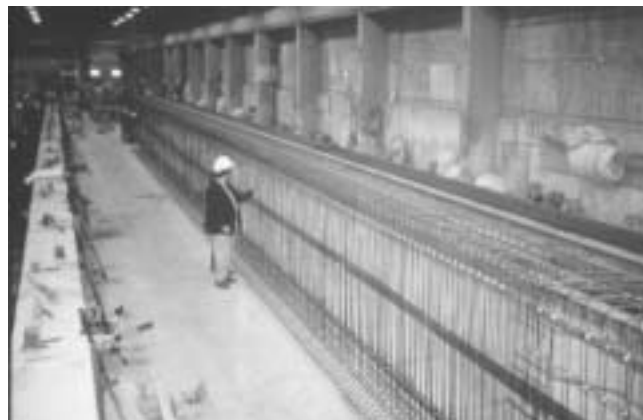
Fig. 1.2—Construction of the FRP prestressed girders for the Taylor Bridge in Headingly, Manitoba, Canada.
