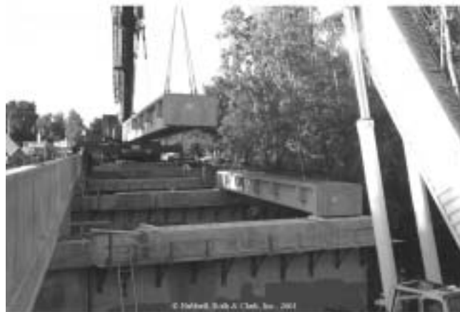
Fig. 1.4—Erection of the Bridge Street Bridge, Southfield, Mich. (Courtesy of HRC Consulting Engineers, Inc., Mich.)
